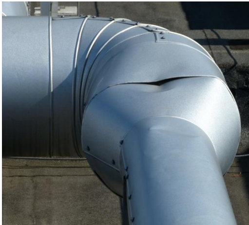
External application - The result of foot traffic and no inspection and maintenance!
