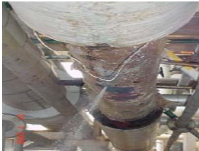
The extreme result of water penetration, product escapes!
