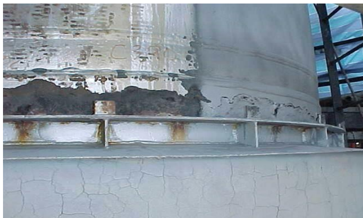
Effects of water penetration at vessel stiffener
